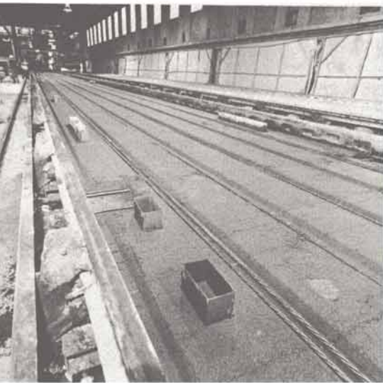
Before hollow-core slabs are poured, tension cables and penetration forms are positioned.
