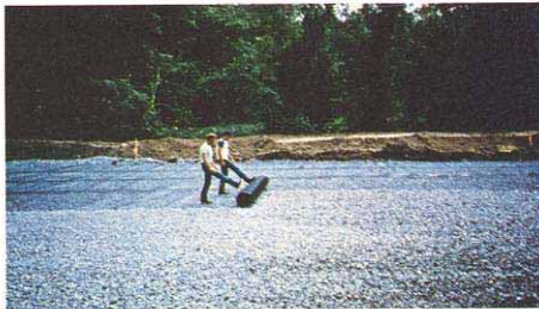
Geogrid material is unrolled on aggregate in preparation for next layer of aggregate.
