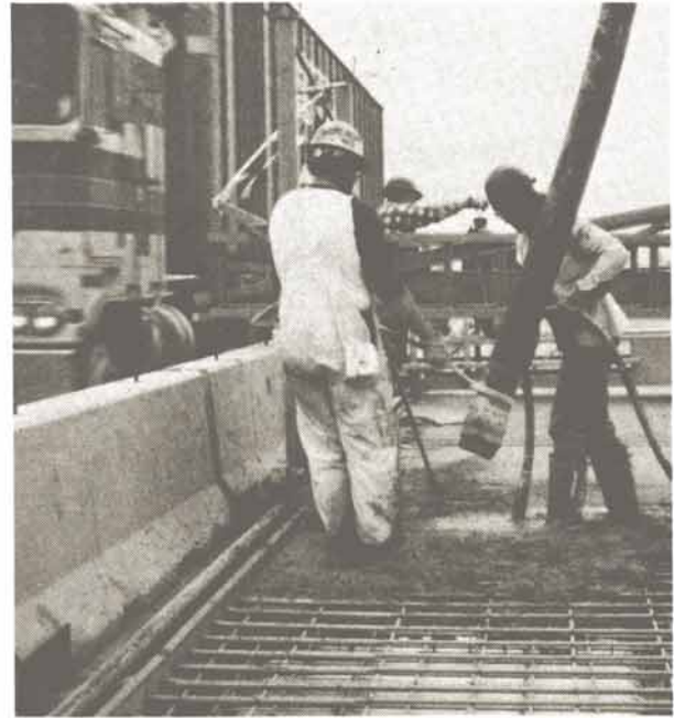
Workers utilizing flexible hose on boom are able to place the concrete where it is needed.
