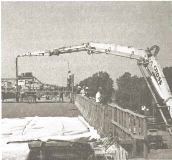
Easy access is provided by pumping concrete up to bridge deck without impeding flow of traffic in opposite direction.
