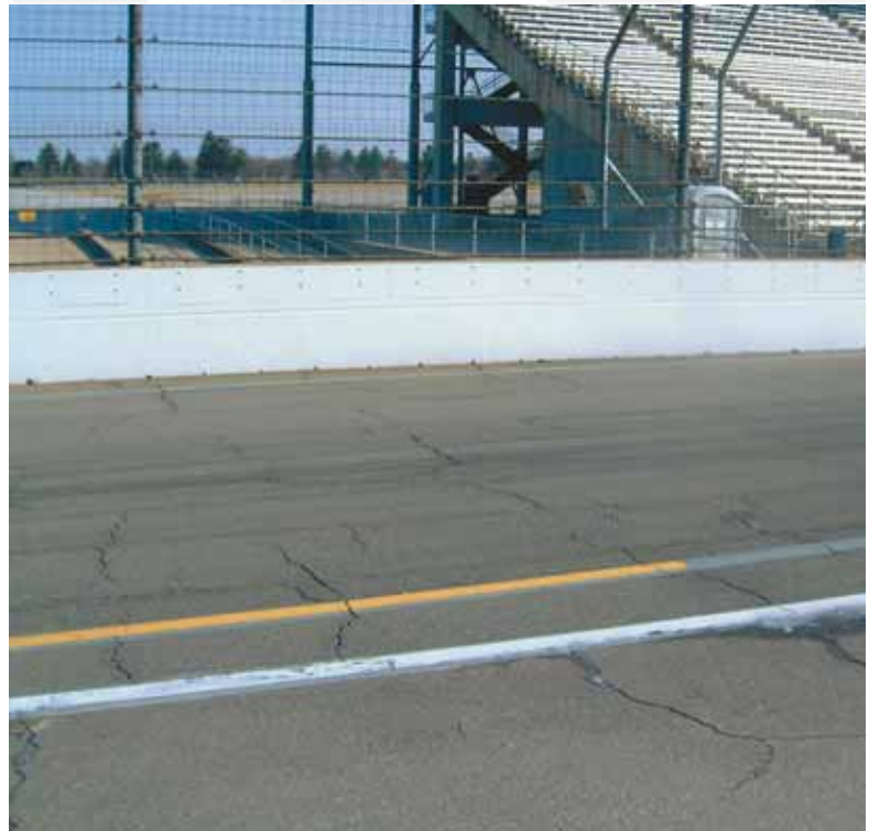
The old track suffered from surface and reflective cracking.
