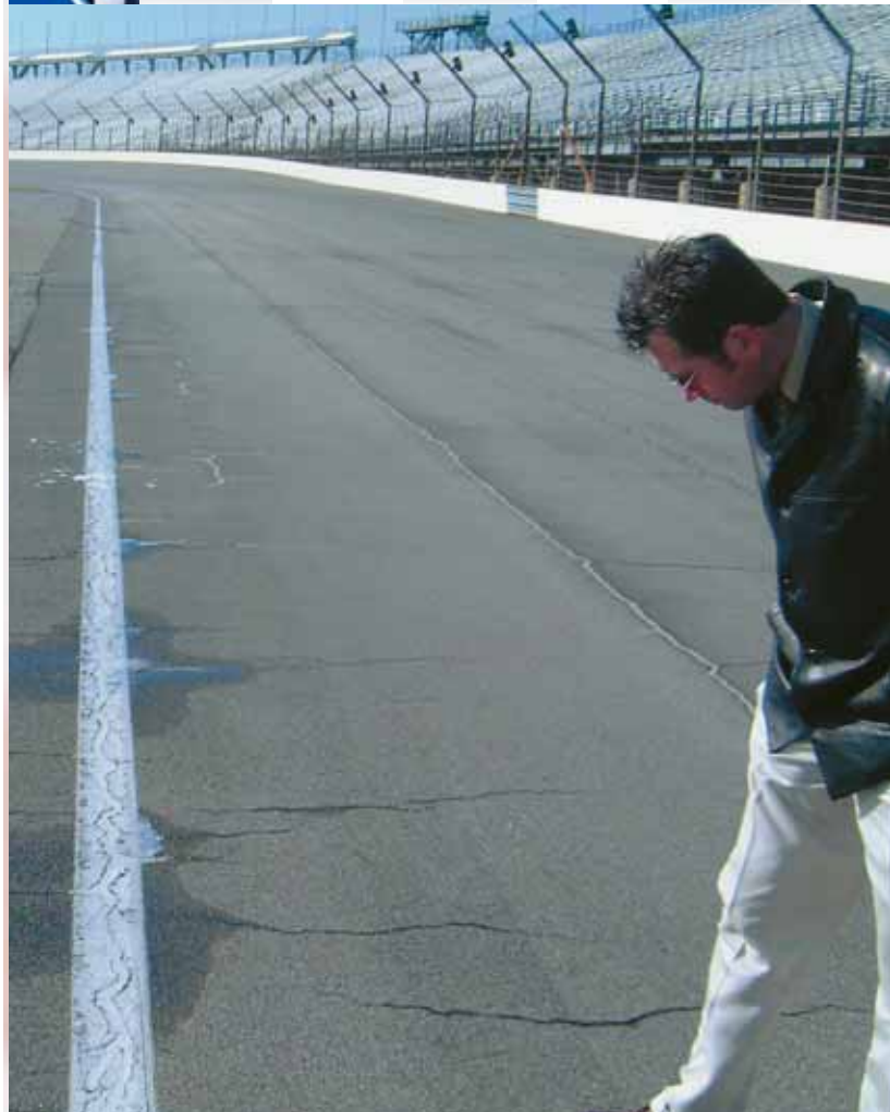
Kevin Forbes, Director of Engineering and Construction at the Indianapolis Motor Speedway, examines cracks in the pavement prior to paving.
