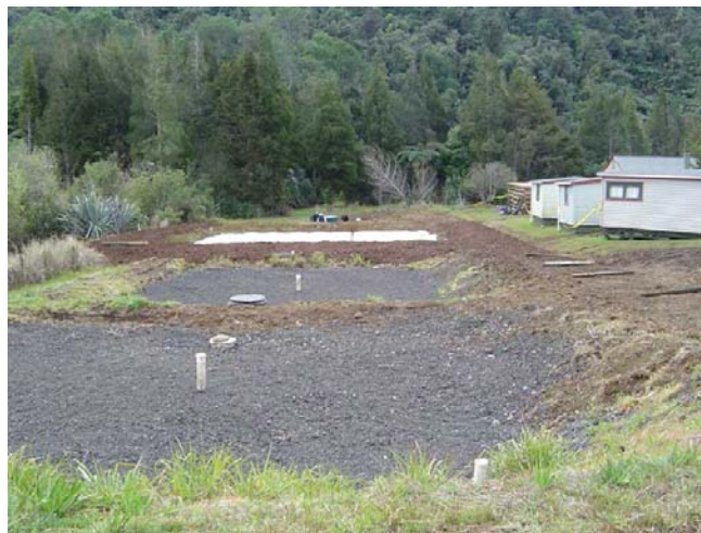
Figure 3: Waipoua Forest Filter beds
