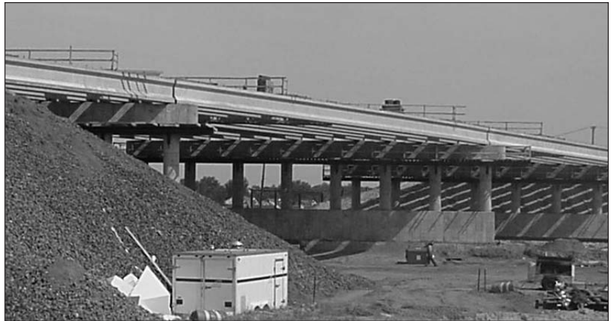
Tons of ACBF slag help provide a cost-effective foundation as Michigan’s M-63 suspended roadway is replaced.
