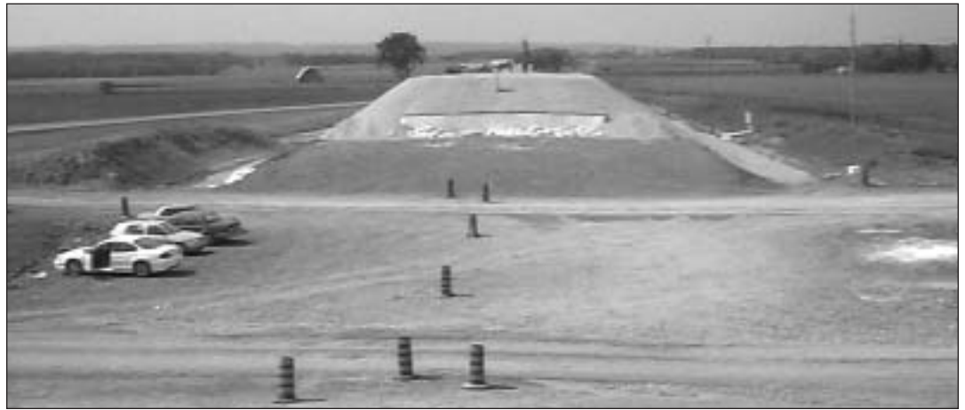
Bridge abutment layers of regular granular fill, Styrofoam® and lightweight expanded slag on top.
