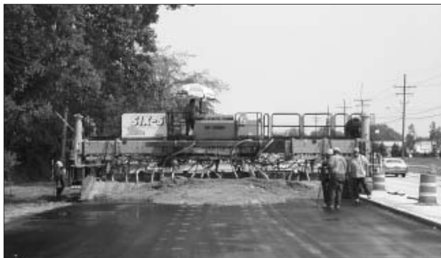
Placement of concrete, including Blast Furnace Slag, supplied by Edu. C. Levy Co., on Merriman Road in Westland, Michigan.
